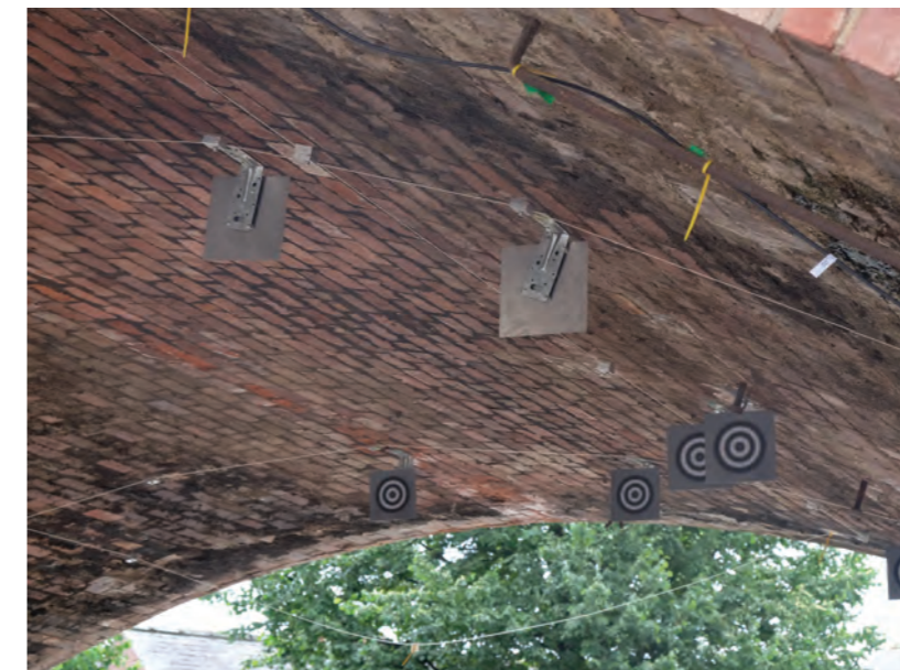
An arch instrumented with FBG cables and photogrammetry targets in the viaduct
