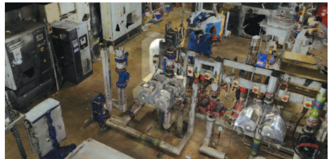
Figure 1: Snapshot of BIM Model of IfM Plant Room from ContextCapture modelling software by Bentley Systems
