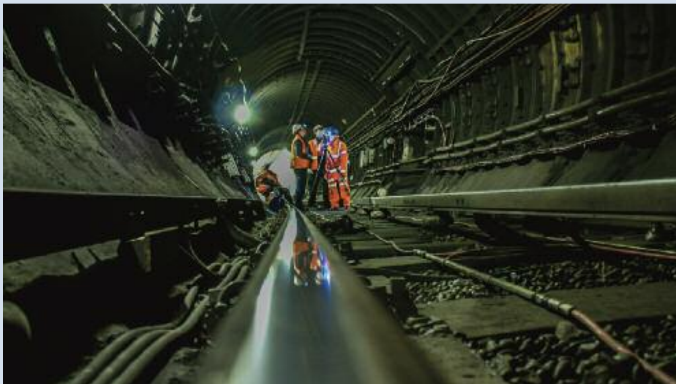
CSIC researchers with engineers from Tubelines surveying the tunnel geometry, feeding into London Underground's overall maintenance strategies
