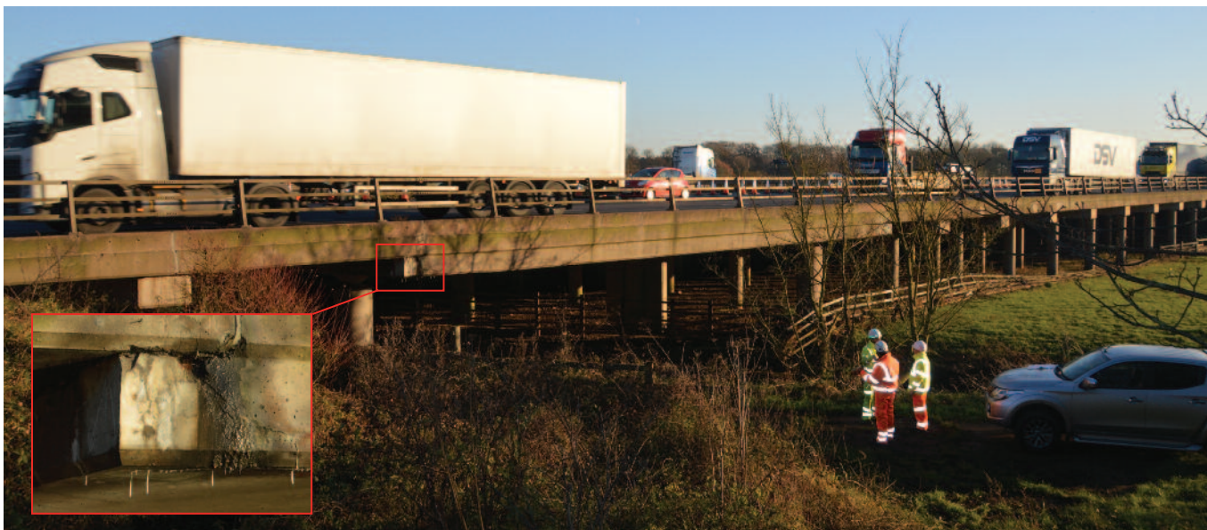
The M6 motorway bridge that crosses the Penk River in Staffordshire and (inset) diagonal cracking and moisture accumulation in the deteriorating half-joint connection of the bridge
