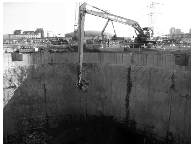
Figure 6. Excavation in front of 1.2 m thick pre-installed diaphragm walls for Crossrail's 30 m dia. and 44 m deep TBM launch shaft at Limmo Peninsula (SBE construction)
