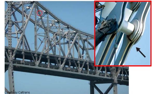
Fatigue (Bay Bridge in CA, 2009)
