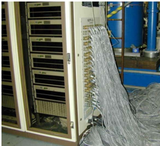
Cabling & instrumentation for 400 wired strain sensors
