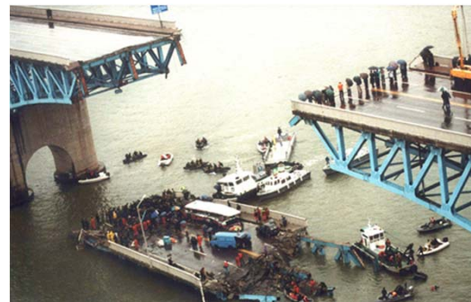
Sung-su bridge collapse in Korea (1994)
