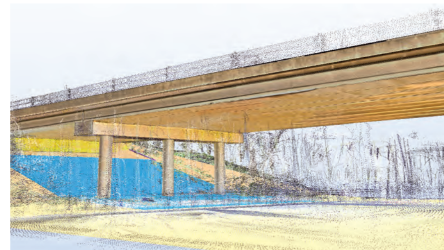
Fully-textured, real size as-is bridge model based on point cloud and high resolution imagery which allows for remote inspection using HoloLens
