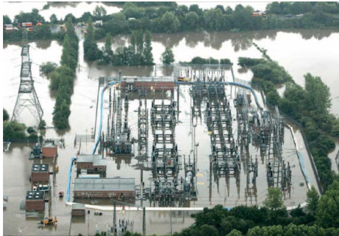
Flooded electricity sub-station UK 2007
