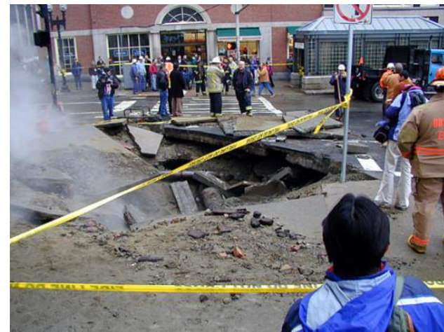
Burst water main Boston 2003
