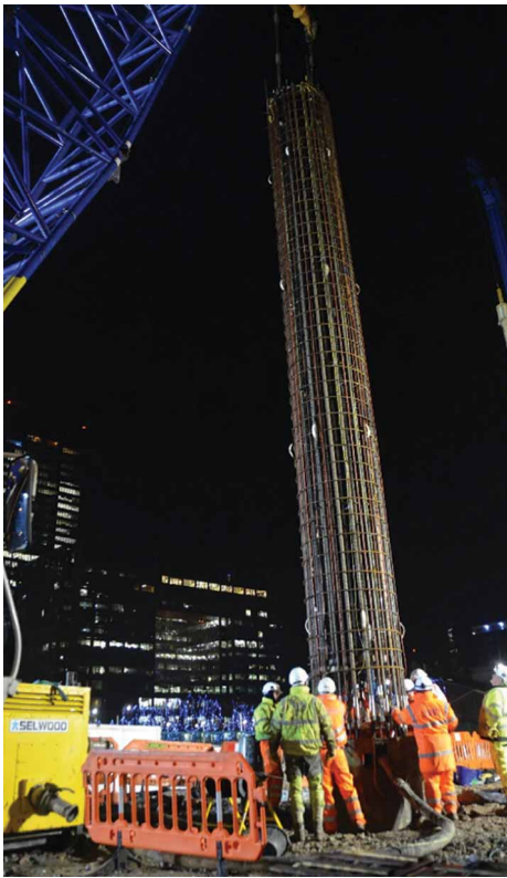
Figure 2: Lowering the cage segment. Engineers have pre-instrumented the rebar cage of a pile about to be constructed. The fibre optic sensors (two are deployed, one for temperature measurement and one for strain measurement) are attached to the steel rebar in a mesh pattern, allowing strain and temperature to be measured at multiple points in a 2D array surrounding the pile itself.
