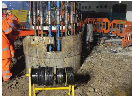
Figure 3: Rebar and sensor network in place. The rebar cage is now in place in the excavated pile cavity. It is now ready for the pouring of concrete which will fully surround the sensors attached to the rebar, which will then become part of the completed foundation structure.
